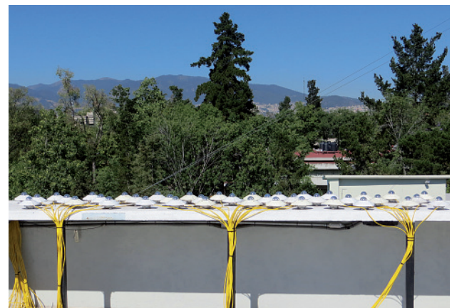
CMP 11 field pyranometers for AWS being calibrated at UNAM
