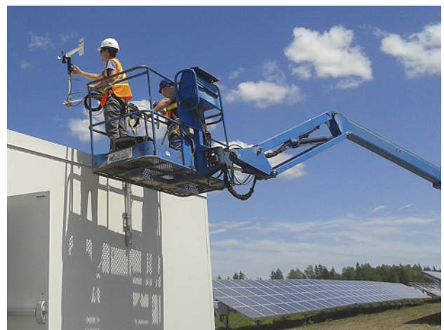
On various sites, services including installation, commissioning, and maintenance are handled through Campbell Scientific's Field Services.
